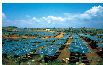
Solar Tracker System
